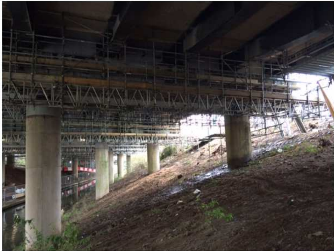
These are the last two sections of 'normal' scaffold being completed underneath the southbound carriageway. There are a couple of special sections still to do; for instance where the viaduct crosses a rail line.
